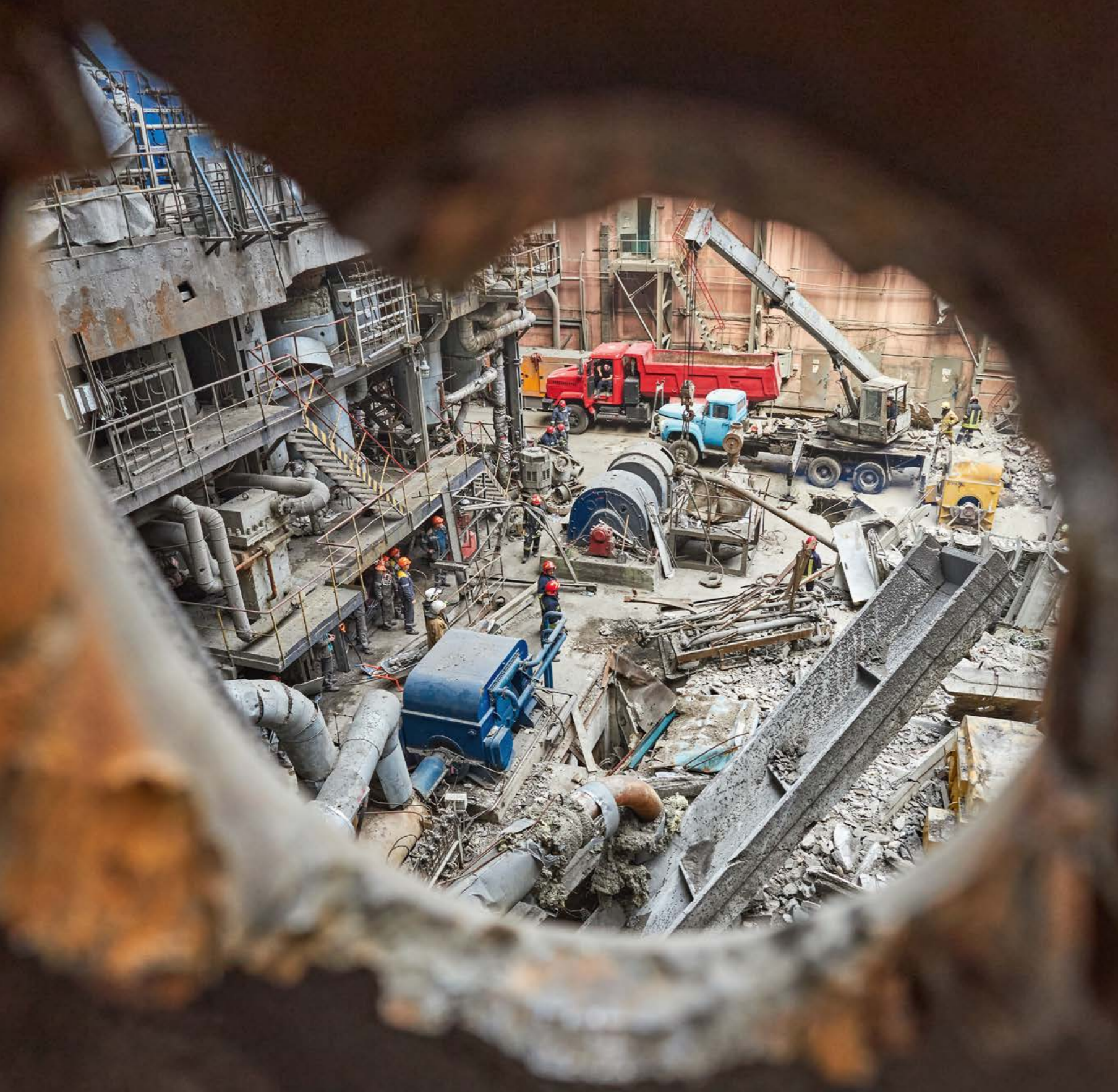
Viewed through a shrapnel hole, engineers breathe life back into a damaged power plant. Serge Serdiukov, 2024
